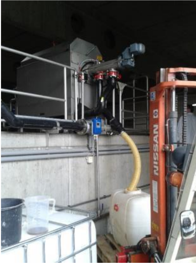
Figure 3: Extraction of biomass from the recirculated fraction of the screen separating ANAMOX biomass (Weissenbacher et al. 2017)
