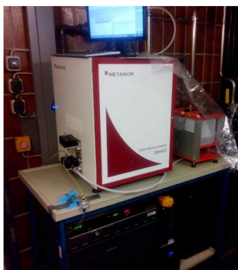
Figure 24: Installed OBA at waterwork
