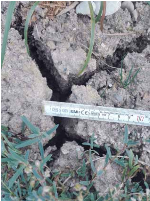
Figure 44. Wide cracks in clay based substrate (Edward Gunn).
