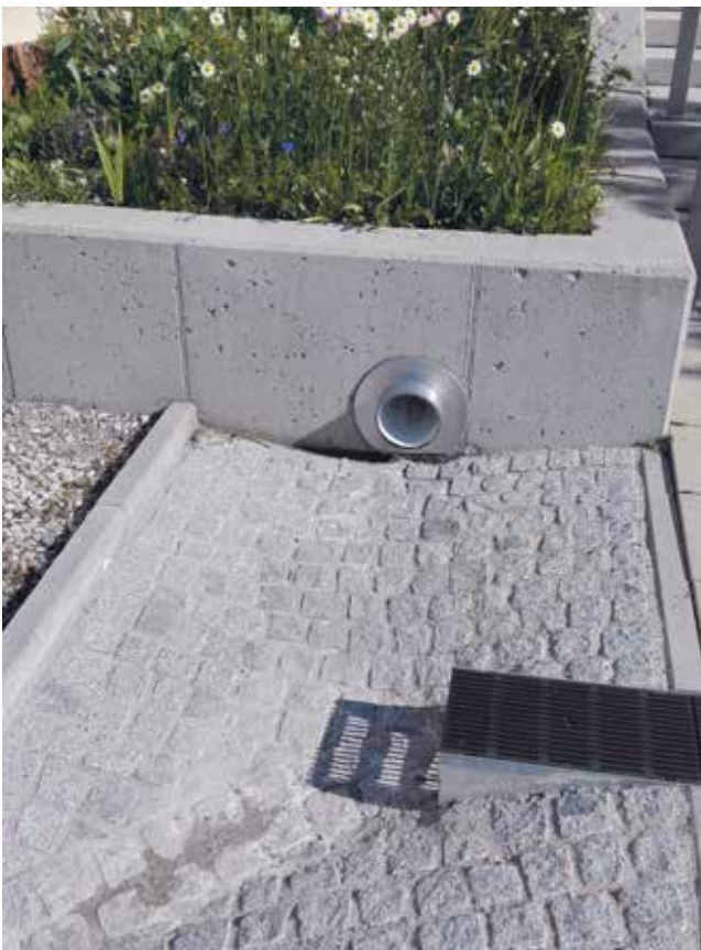
Figure 7. Stage 1 of a stormwater chain: overflow from a stormwater planter flows into a gully, at the University of Innsbruck (Edward Gunn).
