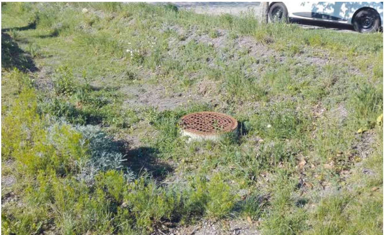
Figure 4. Car park swale collecting surface runoff from a car park at the University of Innsbruck (Edward Gunn).
