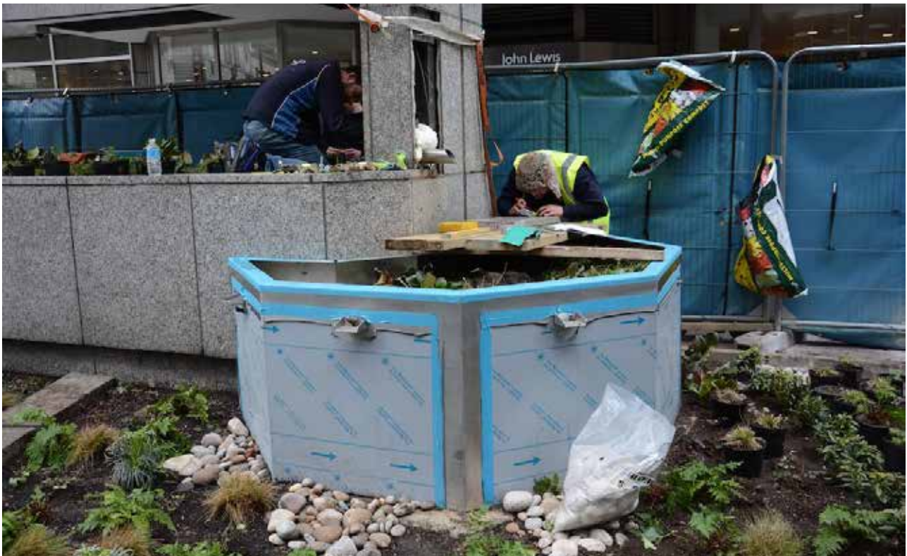
Figure 17. Stormwater planter in John Lewis Group Raingarden, London (Nigel Dunnett & The Landscape Agency).
