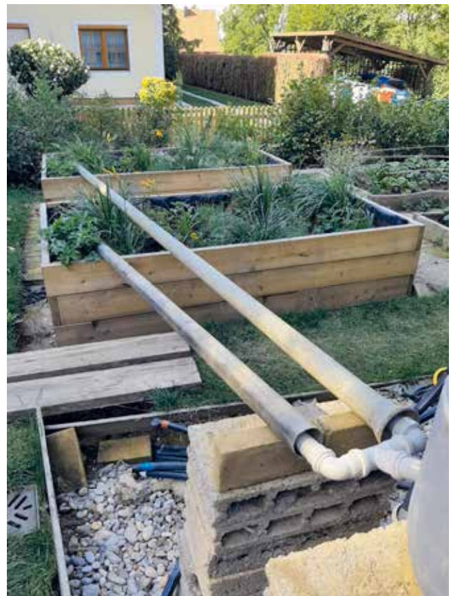
Figure 27. Pipes distributing rainwater equally to each planter (Edward Gunn).
