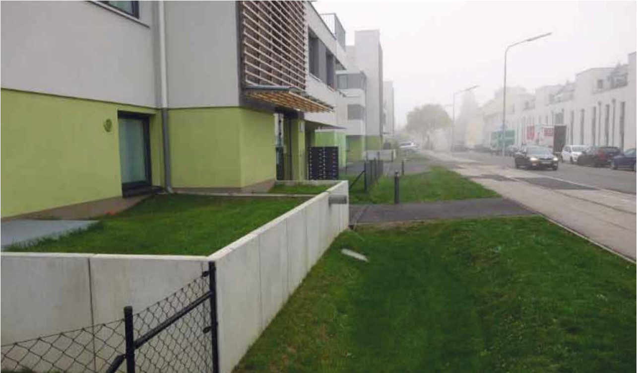
Figure 20, Stormwater chain containing a stormwater planter which can overflow into a grass swale, collecting water from the building down pipe as well as from the road, Wohnpark Süßenbrunnerstraße, Vienna (Karl Grimm).
