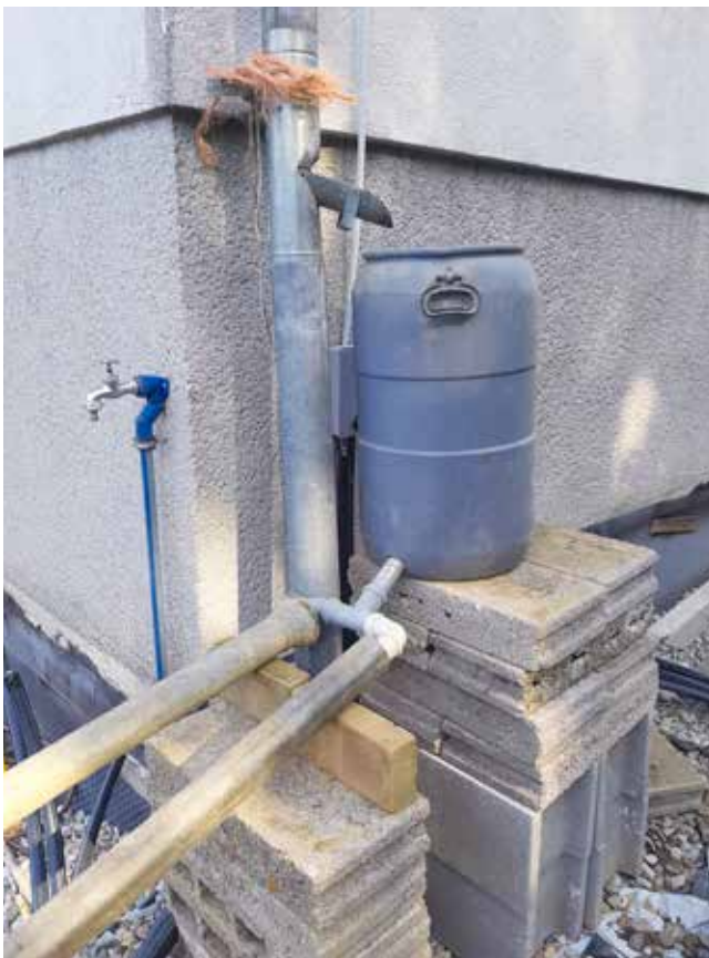
Figure 26. Water barrel collecting rainwater from roof via downpipe (Edward Gunn).
