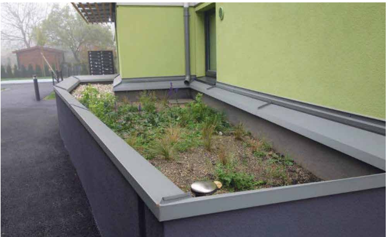
Figure 19. Stormwater planter collecting water from a down pipe, Wohnpark Süßenbrunnerstraße, Vienna (Karl Grimm).
