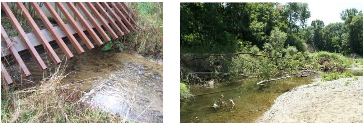
Figure 6: left: bars not reaching the river bed, right: woody debris - habitat for aquatic organism
