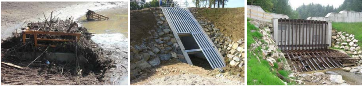
Figure 5: left: blockage of bottom outlet, middle: screen out of removable elements, right: angular screen
