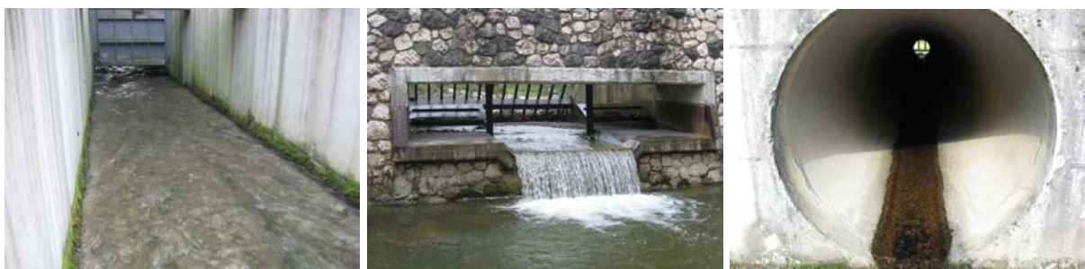
Figure 10: interruption of the continuous water flow, barrier for fish migration, left: unstructured bed of a culvert, middle: large drop heights, right: long, dark section with a small cross-sectional area
