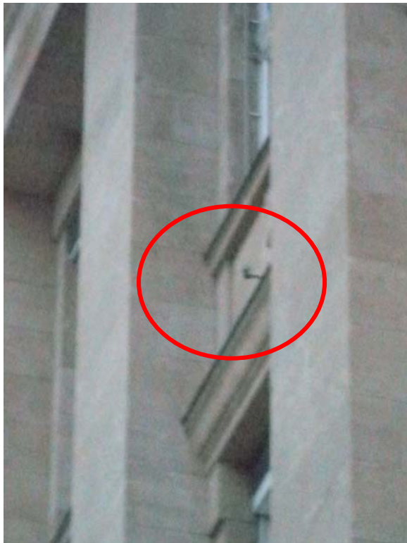
Graph 126: Placement of temperature sensor on west facade
