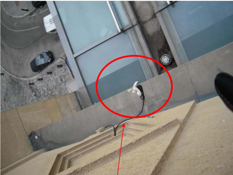
Graph 127: Placement of temperature sensor on east facade
